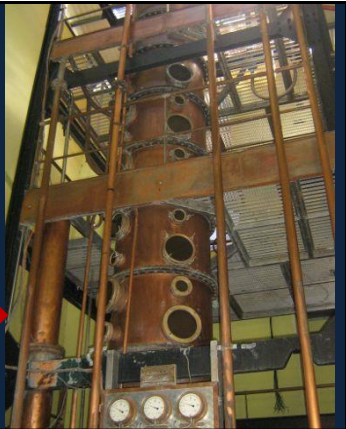
Distillation column at Neisson
