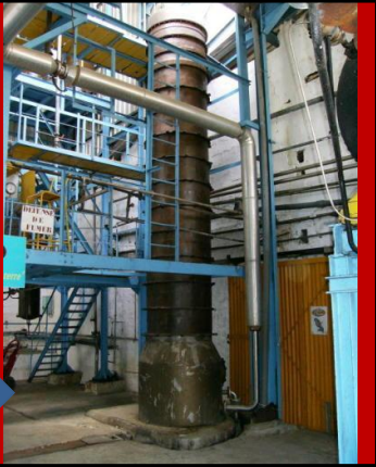
Distillation column at Trois Rivières
